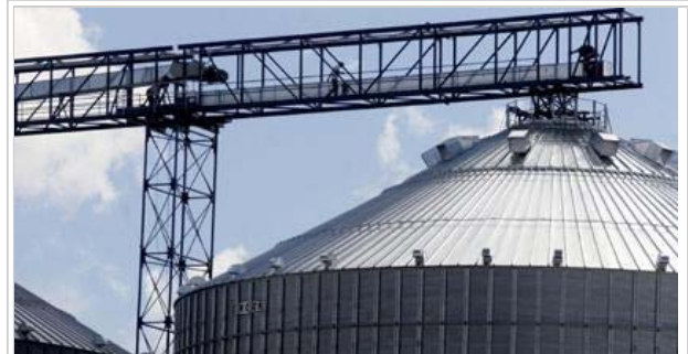
3 September 2010 -- Workers install new corn bins Friday at the Central Indiana Ethanol plant. Photo/Jeff Morehead
